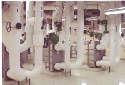
HVAC Process Control
