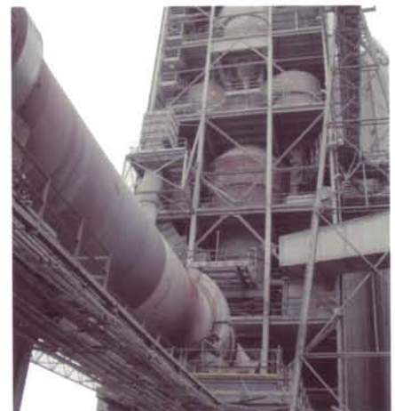
Roller Kiln and Cooling Tower
