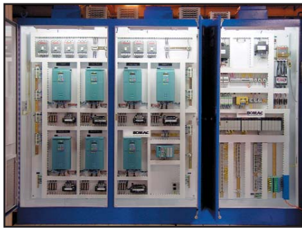
Multi section AC Vector Drive System w/ plc
