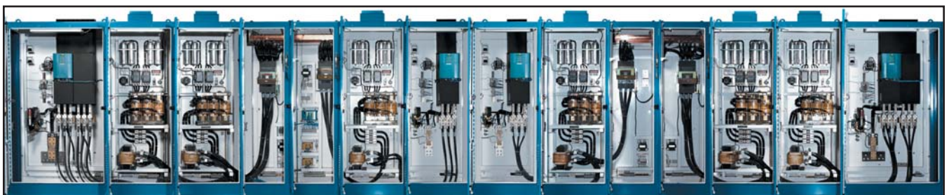
Extrusion Laminating Line DC Drive System
